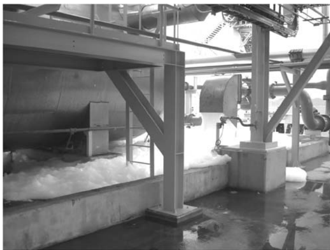
Figure 6.13 Foam fire-fighting fixed system in test operation, installed to operate in the containment basin built to protect spills from pressure vessels. Courtesy J.C. Melchior's personal archives.
