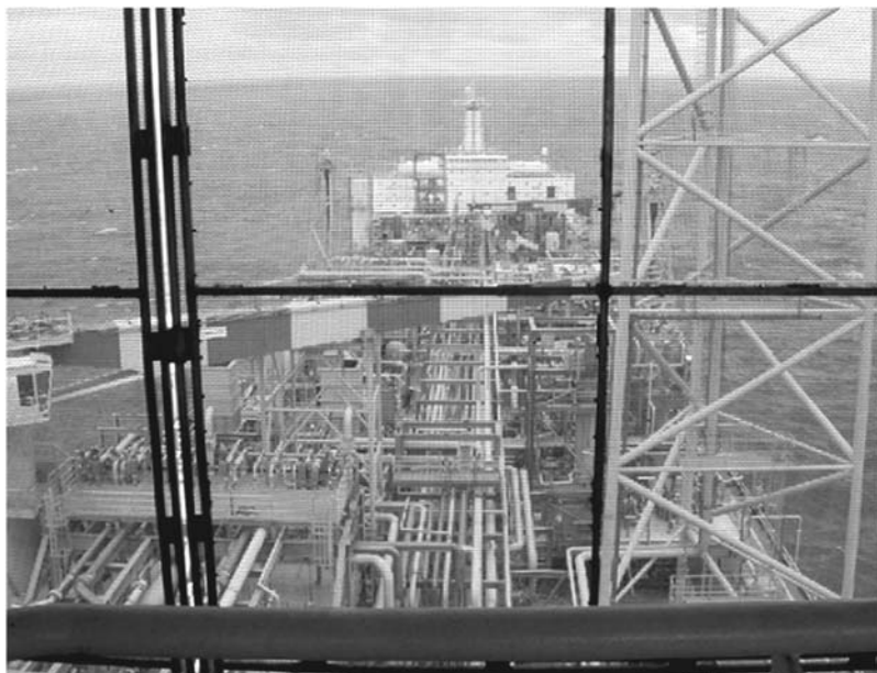
Figure 4.8 Heat dissipation systems in the flare region. Also known as heat shielding, they are made up of panels similar to screens that protect structures and people from excessive heat radiation.
