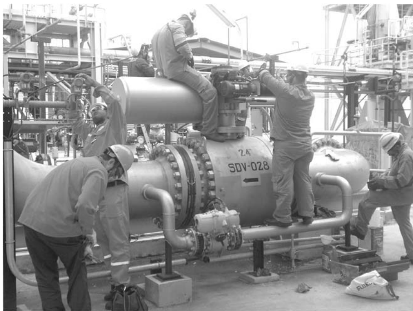
Figure 4.2 SDV during maintenance. SDV, Shutdown valve.
