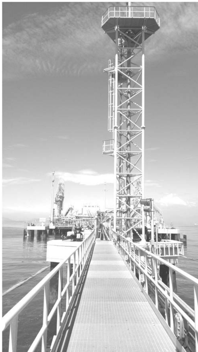
Figure 4.5 Detail of the support structure of an atmospheric vent. The hydrocarbon inventory is safely discarded to the open area in a controlled manner, using natural ventilation and away from sources of ignition.
