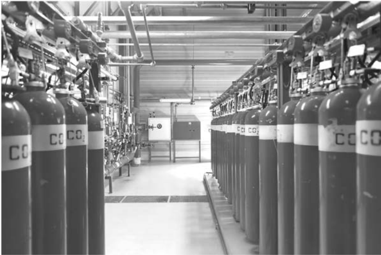
Figure 6.17 CO 2 room with cylinder set of a carbon dioxide fire extinguishing system.
