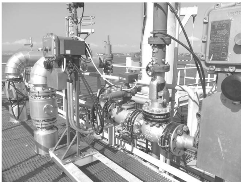
Figure 4.3 Relief and depressurization valve or BDV awaiting maintenance procedure. BDV, Blowdown valve. Courtesy J.C. Melchior's personal archives.
