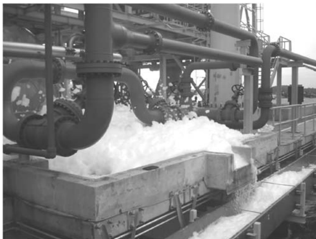
Figure 6.18 Foam flood system test in which the liquefied natural gas spill retaining basin is flooded with foam spilling the excessive volume into the channel connected to the impoundment basin. Courtesy J.C. Melchior's personal file. LNG, Liquefied natural gas.
