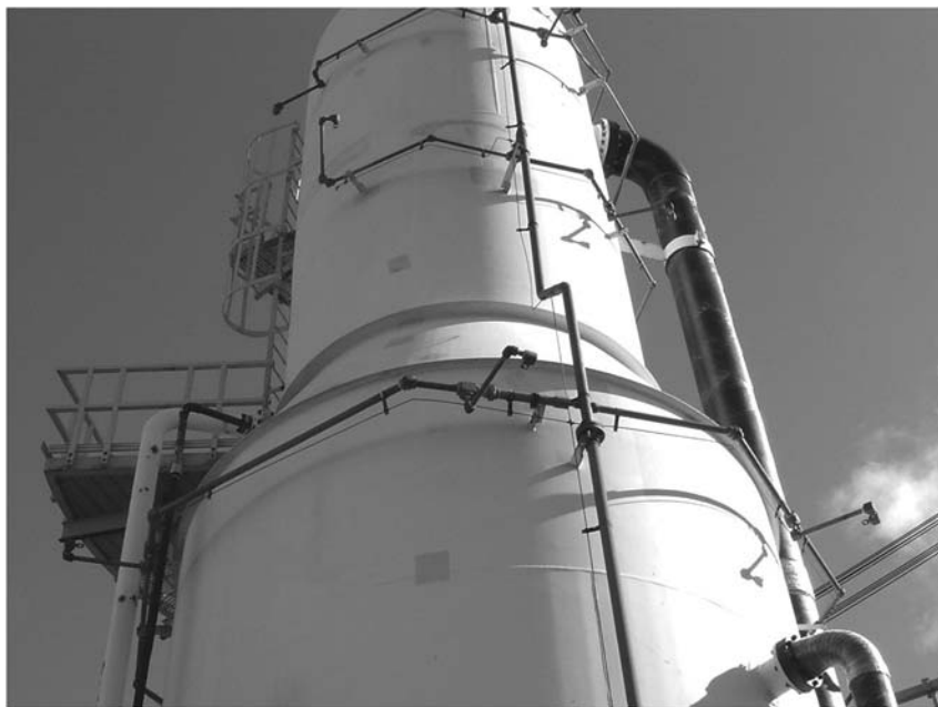
Figure 6.12 Construction and assembly phase of the water spray deluge system. The equipment receives water spray on its external surface as protection against heat from a fire in the adjacent areas.
