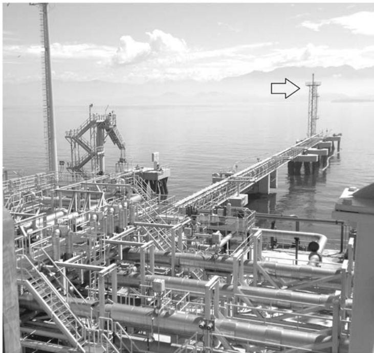
Figure 4.4 Atmospheric vent (indicated by the arrow ) in a process plant: there is no burning. The gas to be discarded is dispersed to the open area exploring the location of the disposal point (free of ignition sources) and exploring the conditions of natural ventilation.
