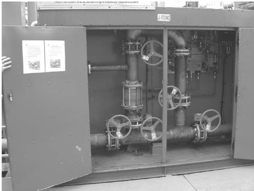
Figure 6.11 Automatic deluge valve assembly installed in a cabinet with identification and operating instructions.
